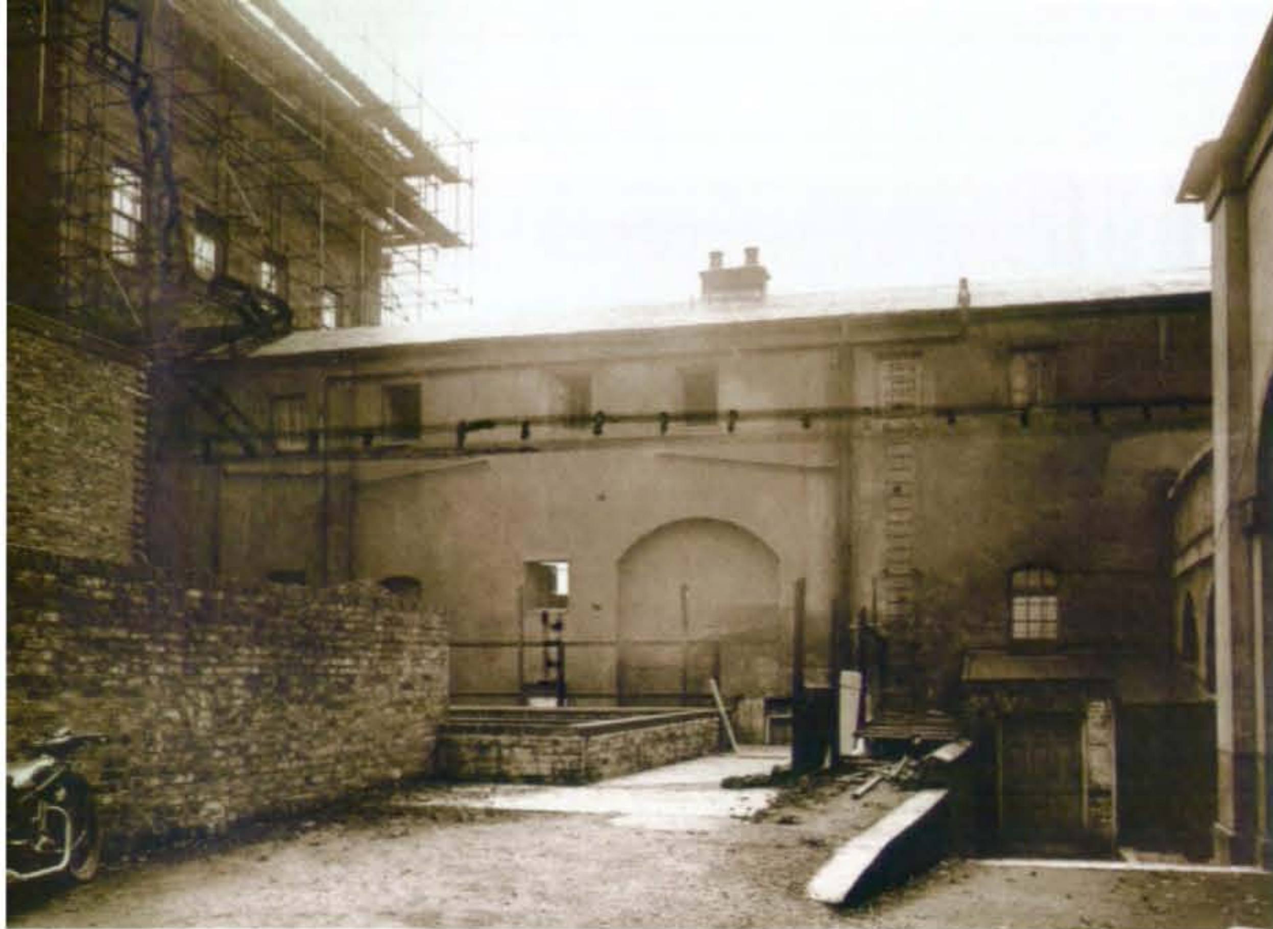
The north side of the southern wing, photographed probably in 1935 when the West Pavilion was under repair. It shows a recessed central arch, perhaps part of Vanbrugh's changes in 1717-24, and also unexecuted plans for external fire escapes.
